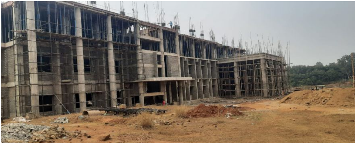
The construction work of new Academic Building is in progress at CUO campus
