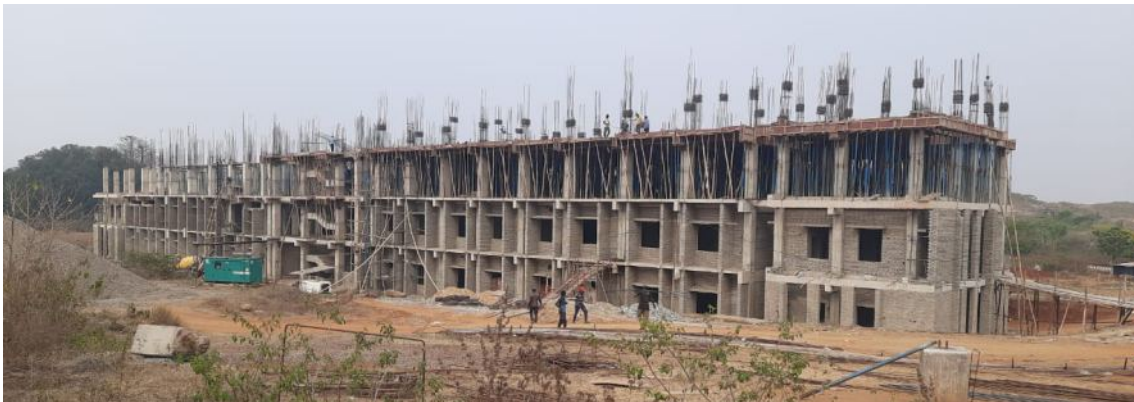
The construction work of new Academic Building is in progress at CUO campus
