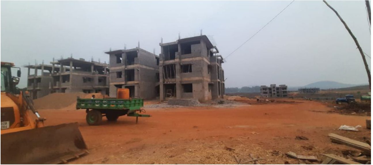
The construction work of staff quarters is in progress at CUO campus
