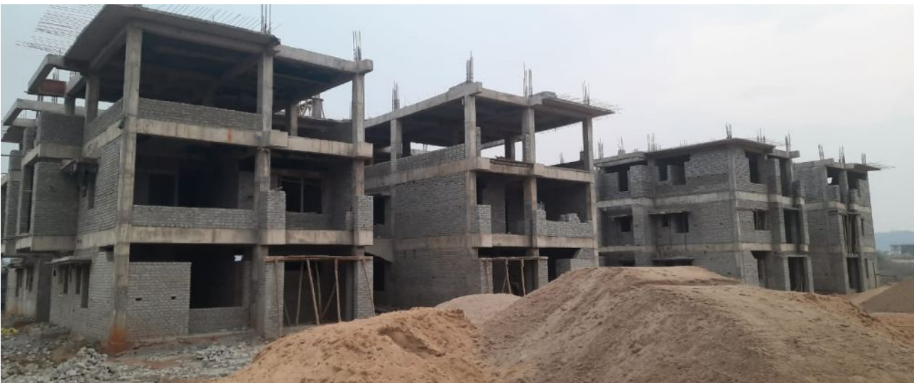
The construction work of staff quarters in in progress at CUO campus
